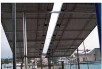
PANEL MOUNTED ABOVE GENERATOR ROOM
