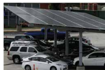
SOLAR PANEL MOUNTED IN THE PARKING AREA
