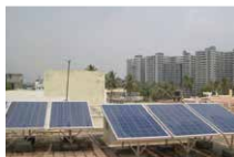
PANEL MOUNTED ABOVE THE TERRACE
